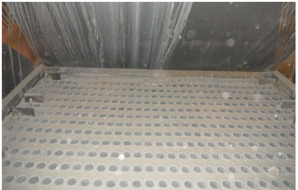
Figure 4: OXYTRON Ceramic Clinker Cooler Inserts were installed at this cement plant to eliminate erosion of the inlet.
